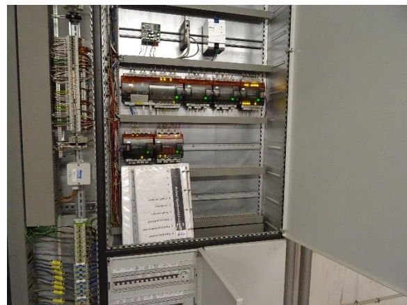
Controller for ventilation
