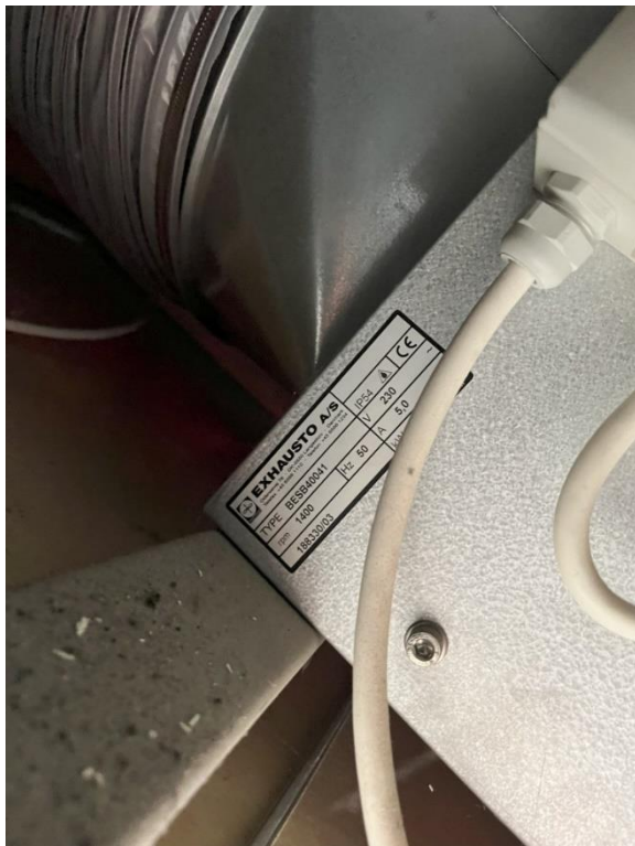
Ventilator over loft
